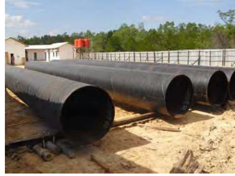
Pipa –pipa diatas rel
